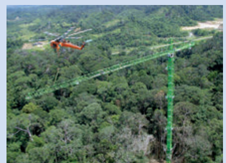
An 80-m-tall canopy crane with a 75-m-long rotating jib in a tropical rainforest, Sarawak, Malaysia
